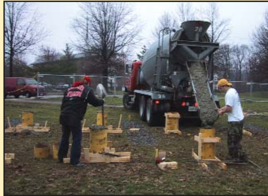
Left: The building process begins: pouring concrete footers on a rainy day in April
